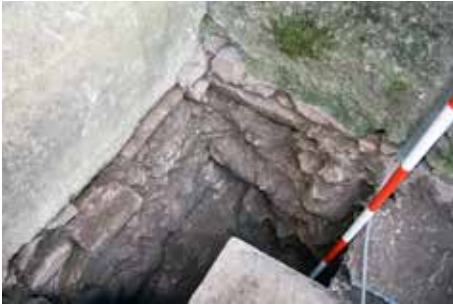
Obr. 6. Sonda S2/11 – cezúra v základovom murive medzi loďou a vežou kostola. Foto A. Balogh. Fig. 6. Test pit S2/11 – gap in the masonry foundations between the nave and the church tower. Photo A. Balogh.
