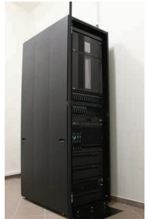
Fig.2: „Heart“ of LIMIS – Rack type box, which contains service station of LIMIS system in Lithuanian Art Museum LIMIS centre. The service station includes 4 Blade type servers, data storage, reserve copying device and source of continuous power supply.
